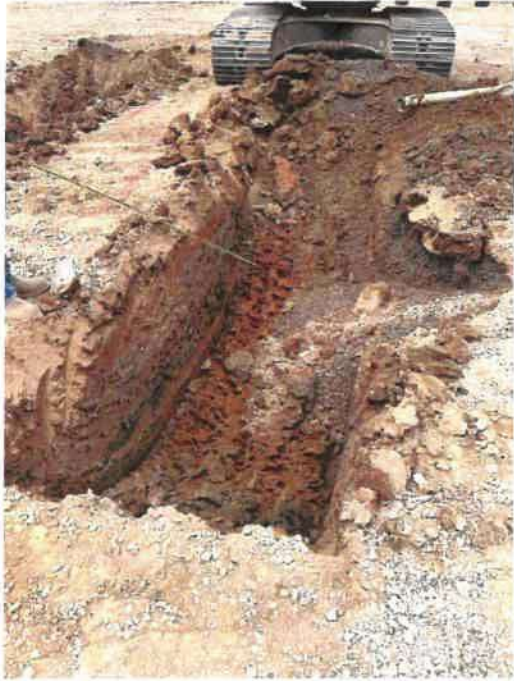
Figure 3: Test Pit Exhibiting Soft Soil Condition
