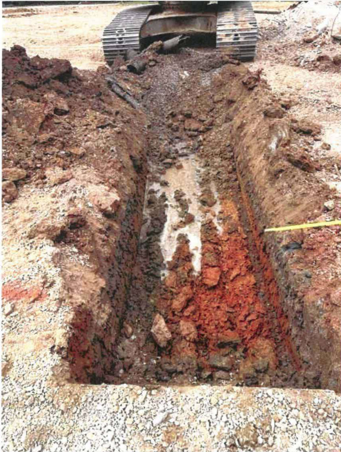
Figure 2: Test Pit Exhibiting Perched Water Condition
