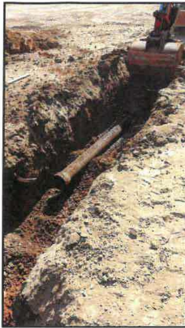
Picture 1: Indicates abandoned utility within footing requiring undercut to suitable soil (column B.5 0.6/0.8)
