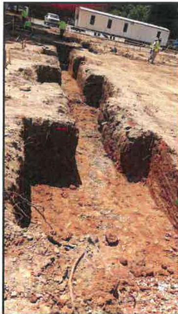
Picture 2: Indicates footings after removal of abandoned utility and undercutting of unsuitable soil (column B.5 0.6/0.8)
