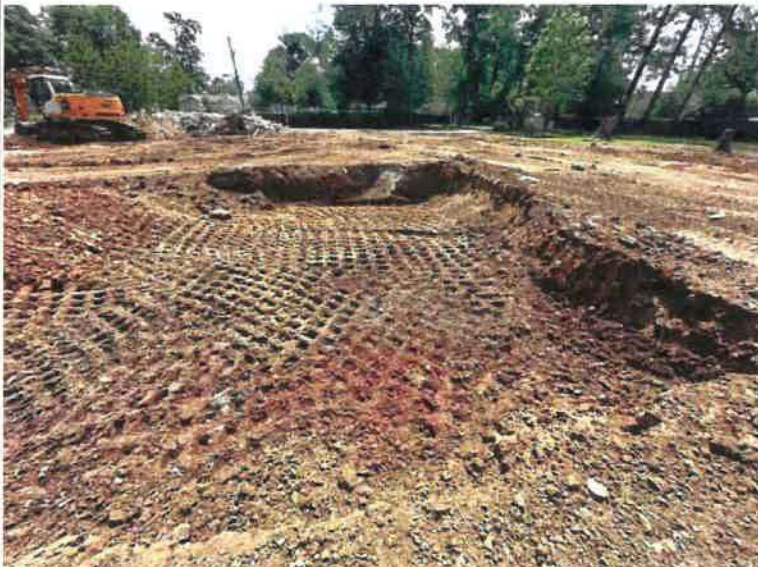
Figure 3: Overall Undercut Area View
