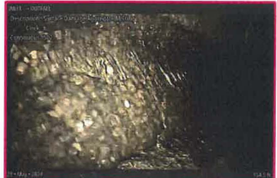
[Grade 4] Surface Damage Aggregate Missing (start) at 154.3 ft, 6 o'clock
