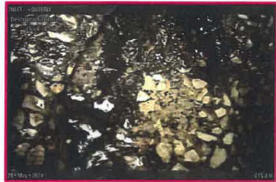
[Grade 4] Broken at 015.8 ft, 4 - 6 o'clock
