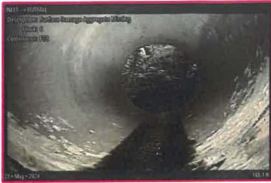
[Grade 4] Surface Damage Aggregate Missing (finish) at 185.1 ft, 6 o'clock
