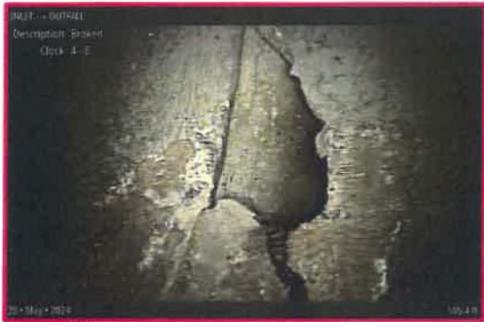
[Grade 4] Broken at 105.4 ft, 4 - 8 o'clock
