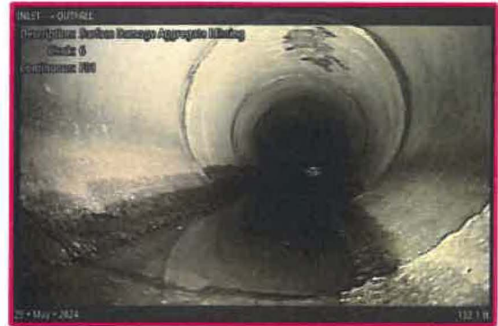
[Grade 4] Surface Damage Aggregate Missing (finish) at 132.1 ft, 6 o'clock
