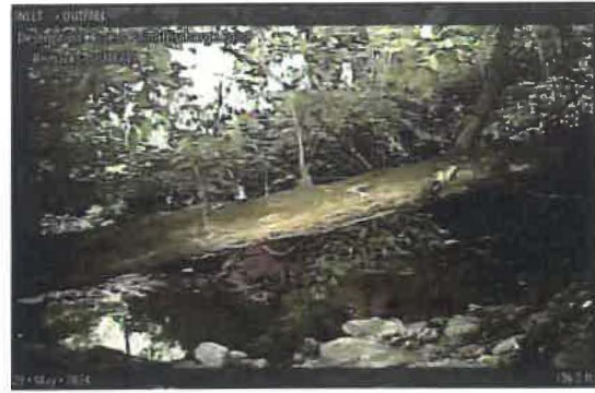
Access Point Discharge Point at 196.0 ft | OUTFALL
