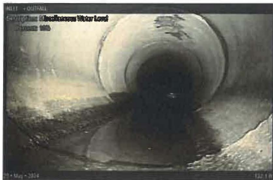
Miscellaneous Water Level at 132.1 ft
