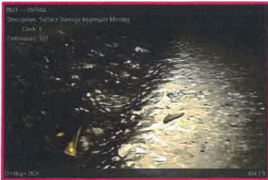
[Grade 4] Surface Damage Aggregate Missing (start) at 000.1 ft, 6 o'clock
